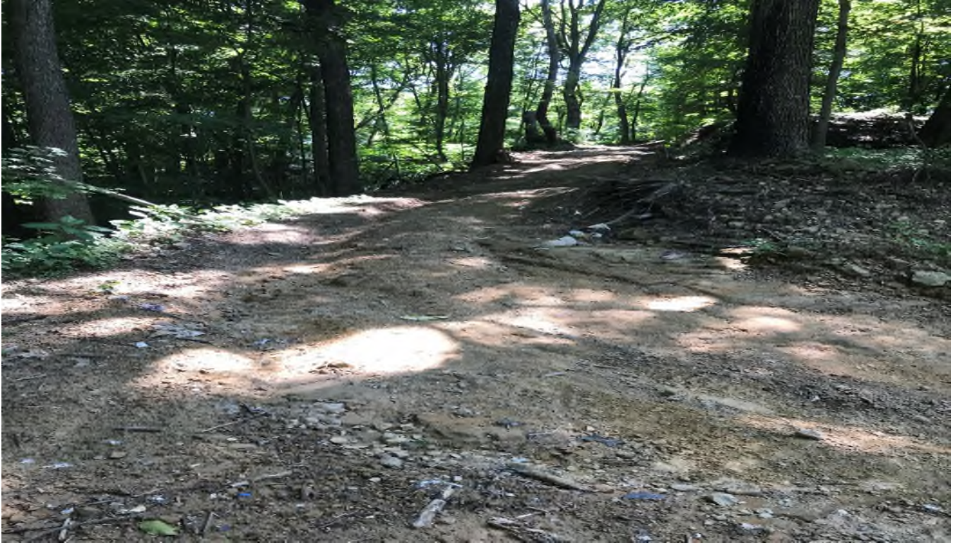
Figure 05 (New land disturbance associated with either new trail construction or widening of an existing trail. Facing uphill toward capped landfill; 37°16'06"N, 82°08'13"W)
