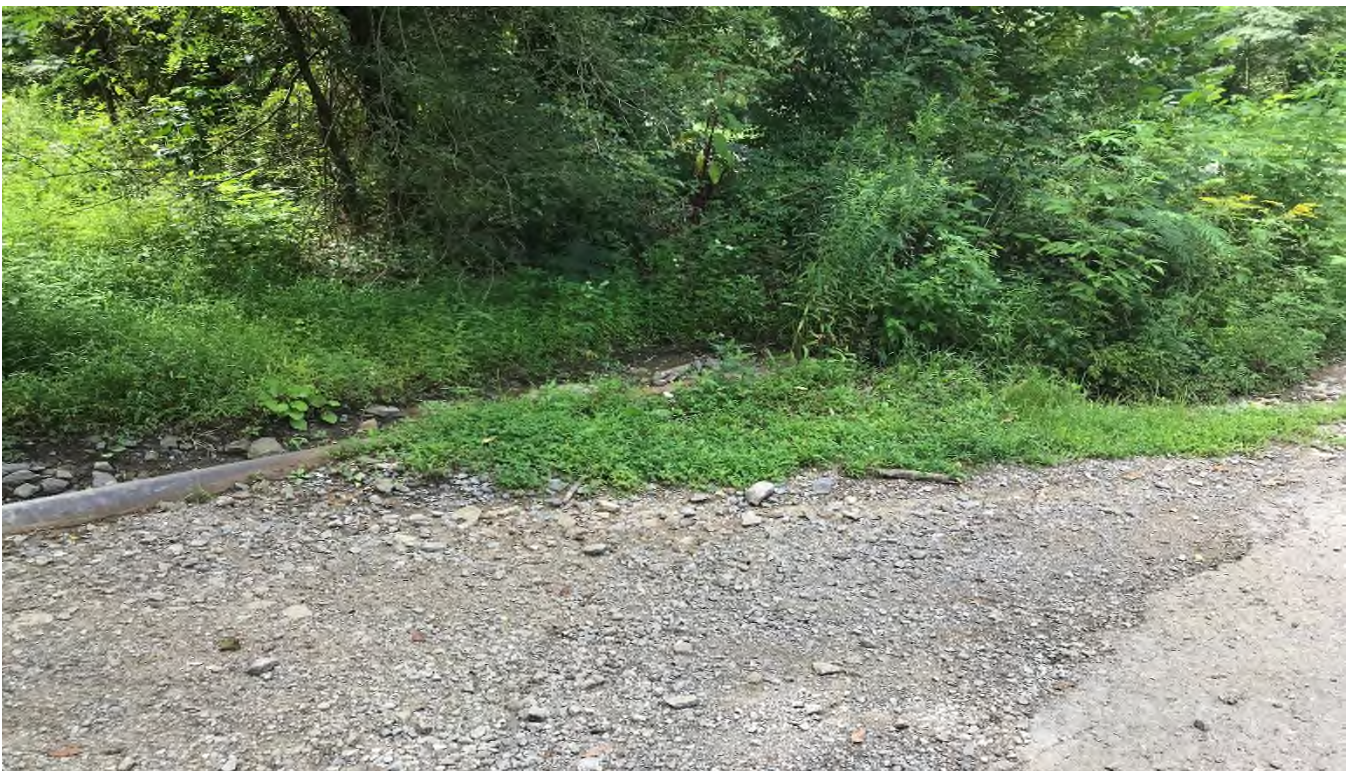
Figure 12 (Concentrated flows from entrance in Figure 11 above bypassing existing culvert, resulting in erosion; 37°16'53"N, 82°06'56"W)
