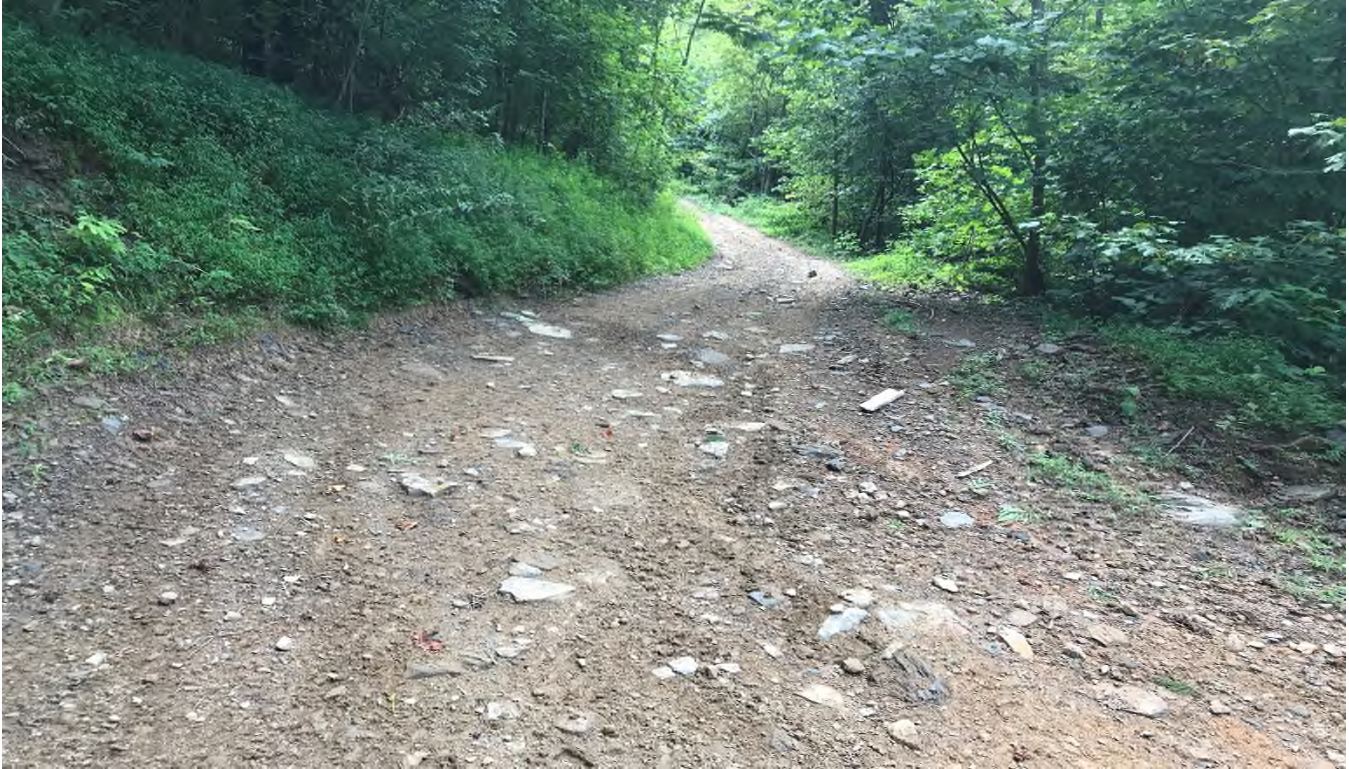
Figure 25 (New land disturbance associated with either new trail construction or widening of an existing trail leading to the area depicted in Figures 23 & 24 above; 37°16'49"N, 82°06'51"W)
