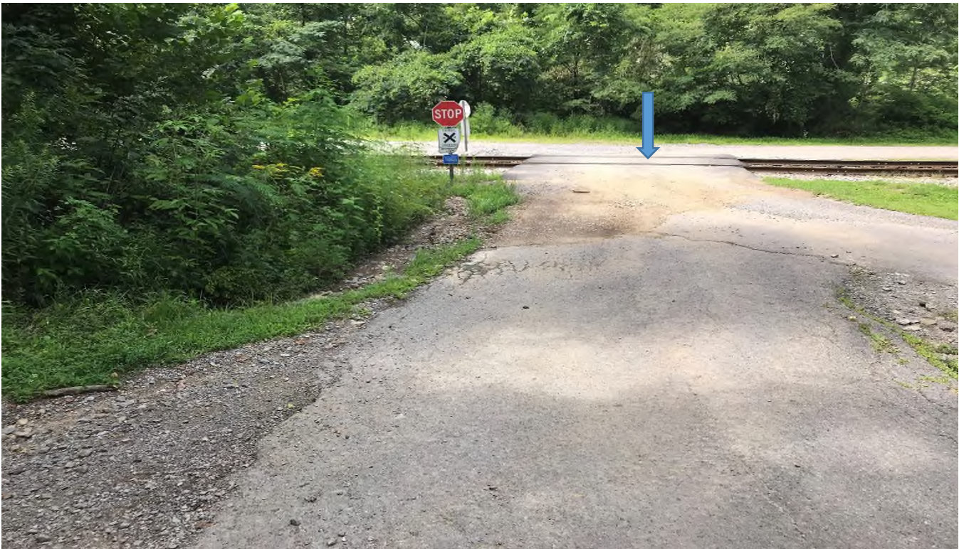
Figure 13 (Residential entrance and rail crossing down gradient of entrance and culvert shown in Figures 11 & 12 above. Sediment deposition in driveway; 37°16'53"N, 82°06'56"W)
