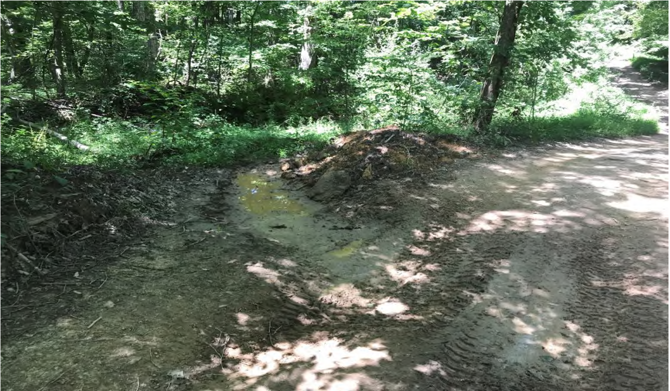
Figure 07 (Window cut on section of trail sending concentrated flows over the slope; 37^{\circ}15'56''\text{N} , 82^{\circ}07'55''\text{W} )
