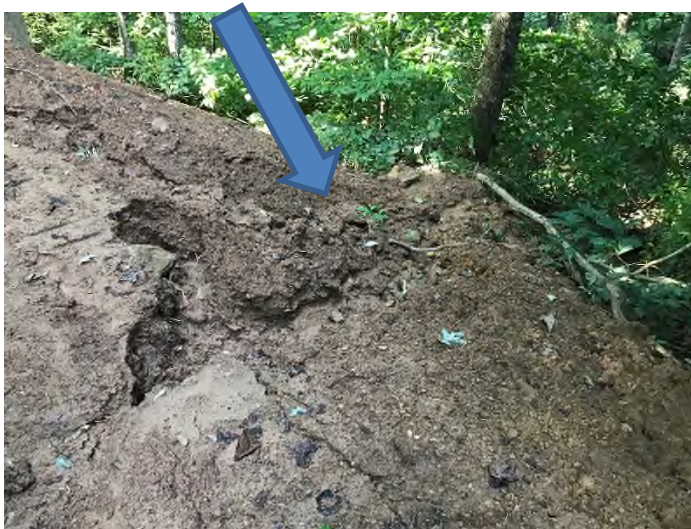
Fig. 15 Description: Concentrated stormwater runoff directed down fill slope and not contained within an adequate slope conveyance resulting in slope erosion and off-site sediment loss
