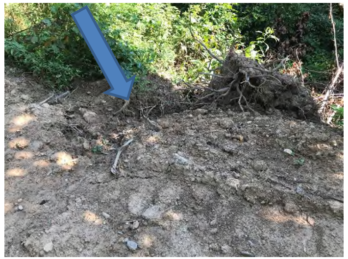
Fig. 16 Description: Concentrated stormwater runoff directed down fill slope and not contained within an adequate slope conveyance resulting in slope erosion and off-site sediment loss
