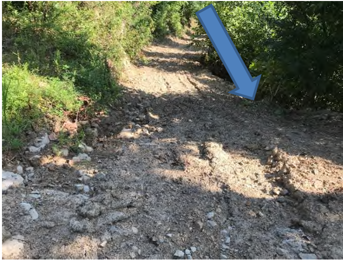
Fig. 13 Description: Concentrated stormwater runoff not directed to an adequate receiving channel or converted to sheet flow
