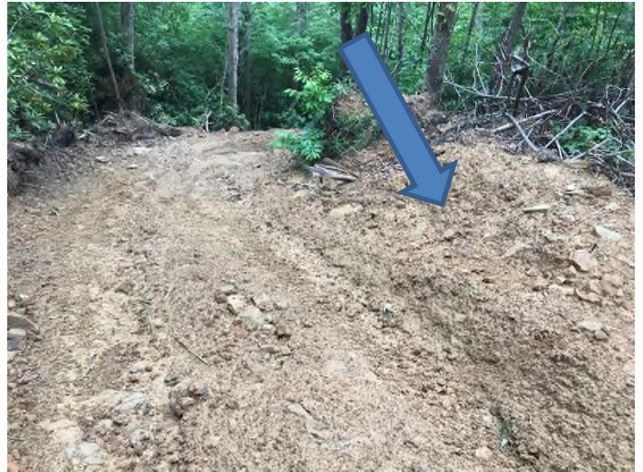
Fig. 6 Description: Stabilization timeframes exceeded
