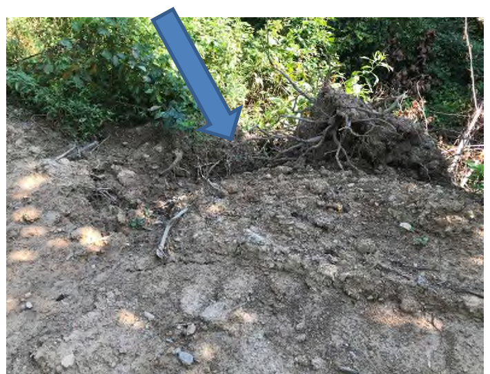
Fig. 10 Description: Fill slope not adequately stabilized to prevent excessive erosion
