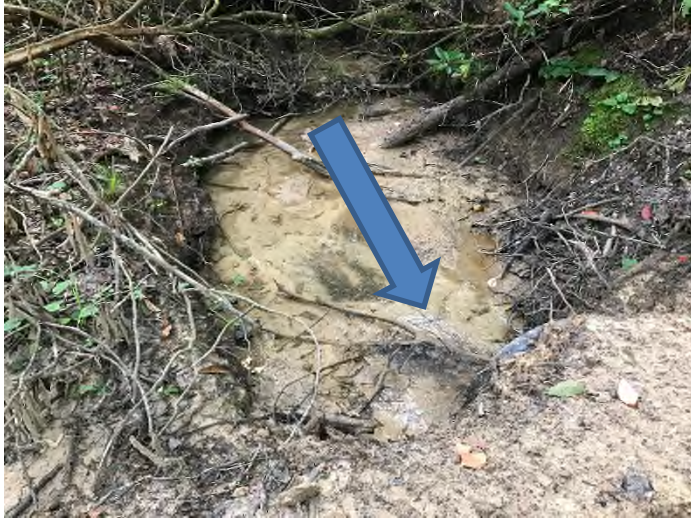
Fig. 17 Description: Lack of outlet protection for culvert installed
