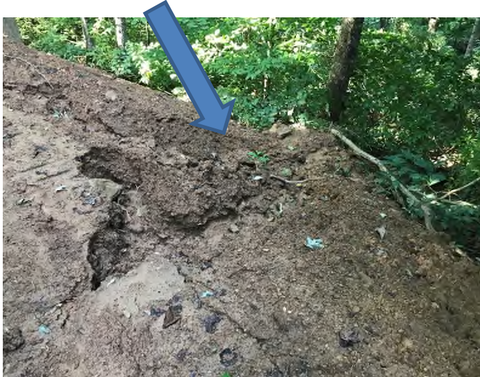
Fig. 9 Description: Fill slope not adequately stabilized to prevent excessive erosion
