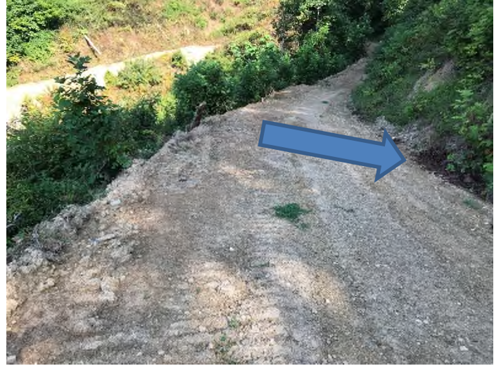
Fig. 18 Description: Cut ditch with no lining and ongoing erosion
