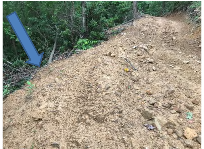
Fig. 12 Description: Fill slopes not designed/constructed in a manner to minimize erosion (Material pushed over slope with no compaction)
