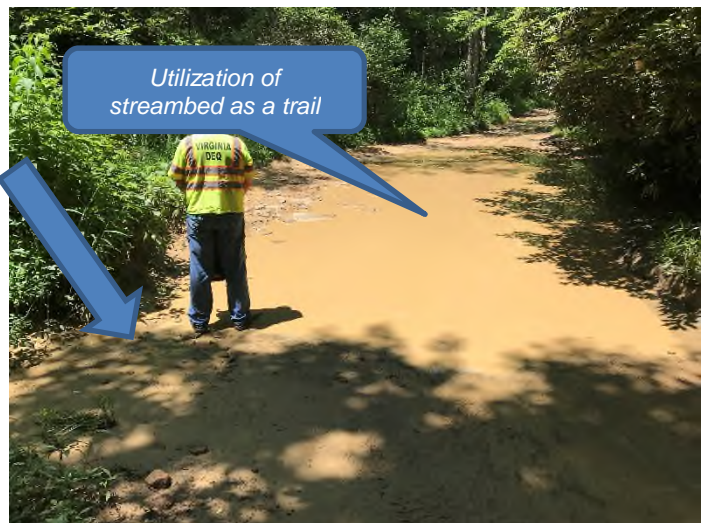
Fig. 32 Description: Sediment impacts to potential jurisdictional stream due to the utilization of the streambed as a trail
