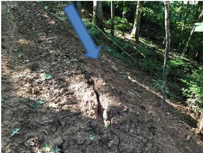
Fig. 11 Description: Fill slopes not designed/constructed in a manner to minimize erosion (Material pushed over slope with no compaction)
