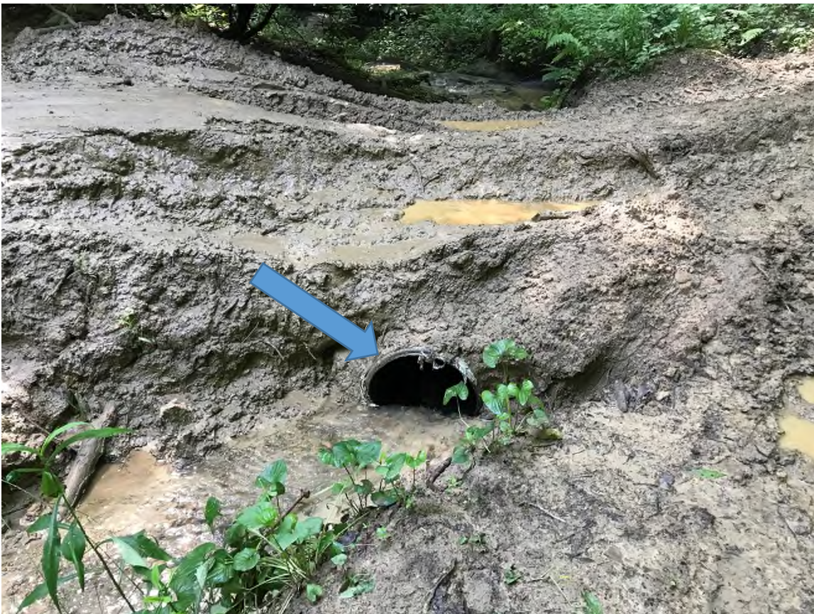
Figure 10 (Inlet of cross pipe at Trail 16 crossing of unnamed tributary of Laurel Fork; 37.29957° , -81.38358° )
